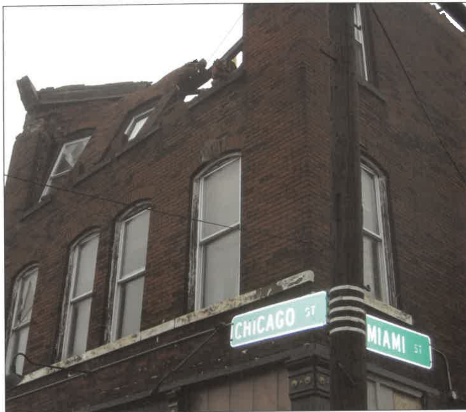
McBride's after the January 30th windstorm damaged the roof and third floor. CLARENCE PICARD PHOTO, 2008
